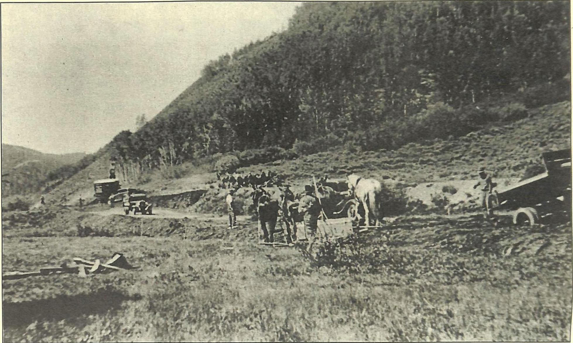
Salt Creek - Smoot Highway under construction, 1934. Inexperienced dump men and truck drivers made it necessary for the contractor to keep a fresno and 4-up on the fills in order to keep a uniform grade as well as spread the material in 6" to 12" layers.
